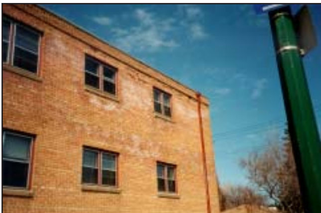
Photo of brick delamination/spalling. Photos supplied courtesy of Retro-Specs Consultants, Ltd. (Kevin Knight)
