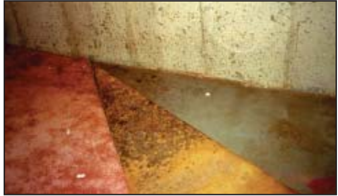
Damp basement areas provide an ideal environment for mold and mildew growth
