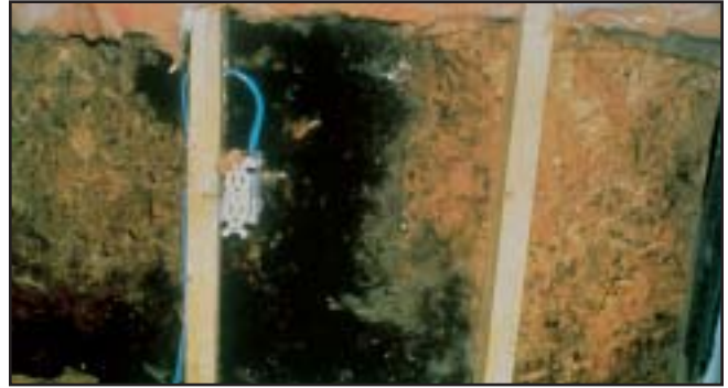
Photo of mold in wall. Photo supplied courtesy of Canadian Home Builders' Association (CHBA) and Canadian Mortgage and Housing Corp. (CMHC)
